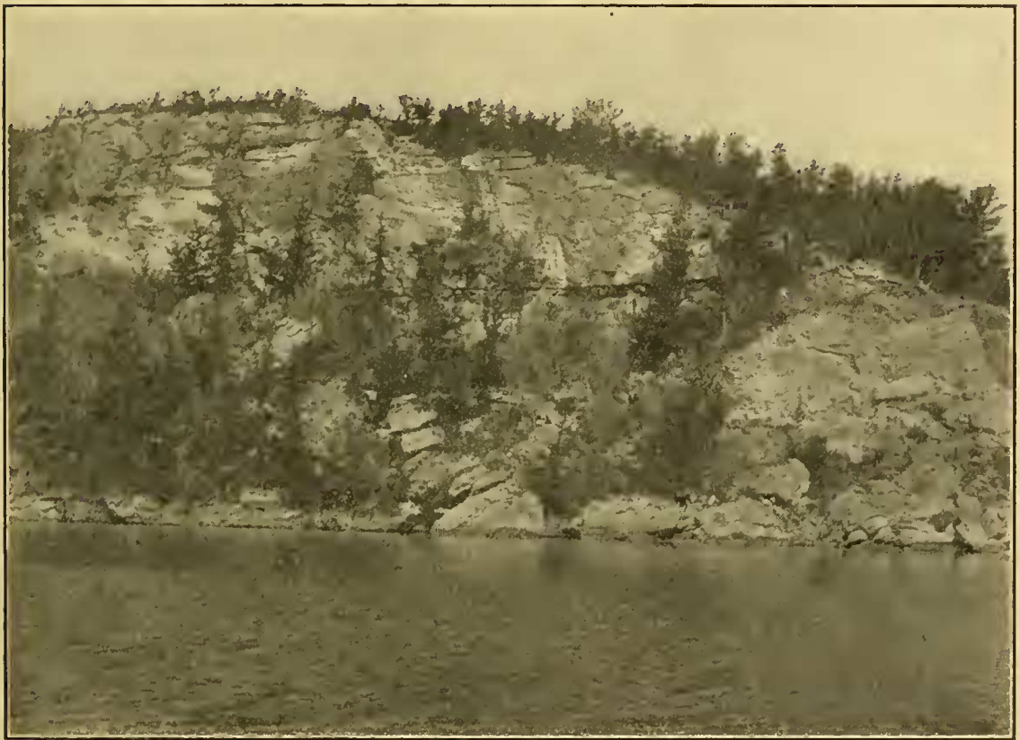
Figure 21.—Abbot's Head, on Harrington Sound, showing the recently fallen masses of rock at base.
